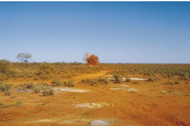
(b) Blasting through the massive calcrete-silcrete with ANFO explosives to excavate pit GCP110, August 1997, view southwest, blast at ~400 m distance. (Photo 45489)
